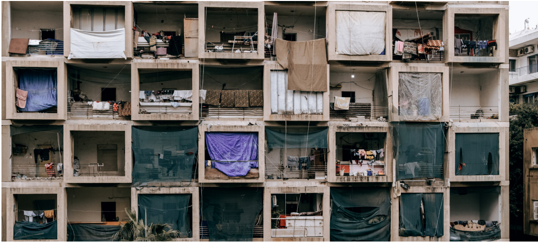
Dilapidated building rented to Syrian refugees in Hamra, Beirut Photo credit: Karine Pierre, reproduced with permission
